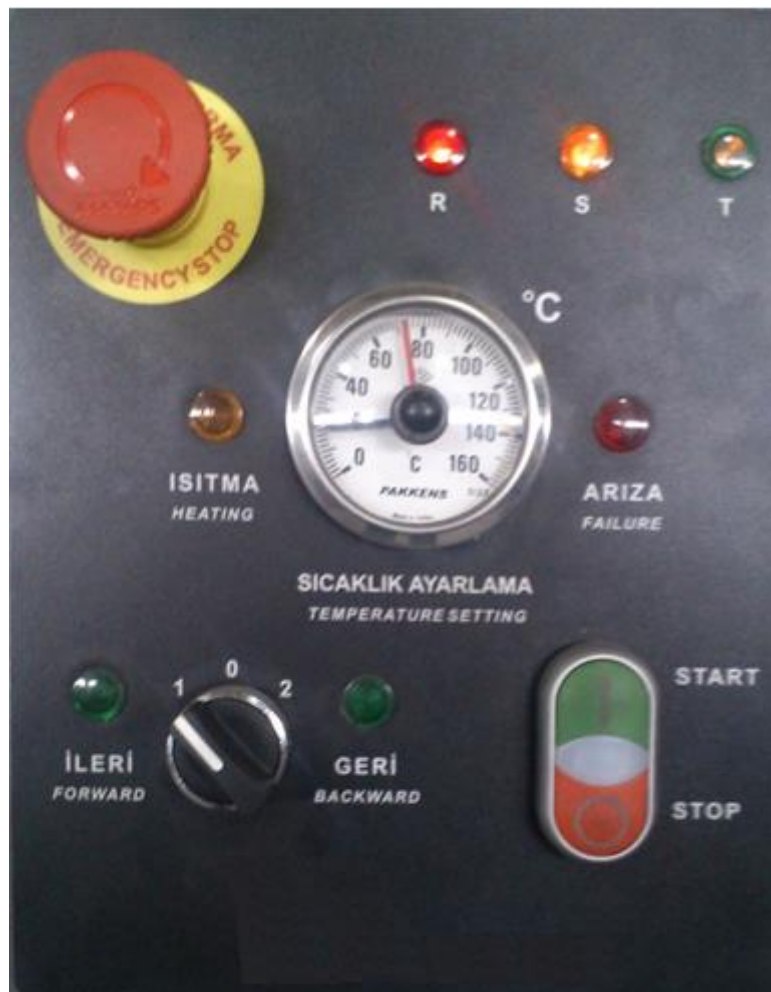
Image – 2 Control Panel
