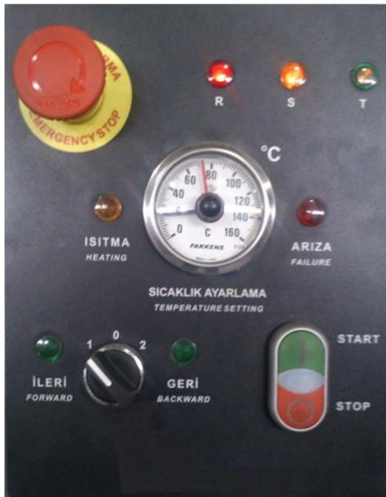
Image – 2 Control Panel
